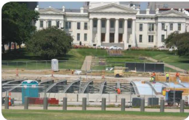
An eight-person crew from Coatings Unlimited, Inc. (CU) was brought in to waterproof the new concrete land bridge over I-44 near the Jefferson National Expansion Memorial park, and, therefore, the St. Louis Arch.
